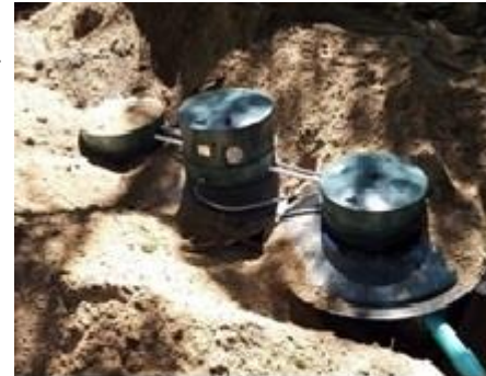
Installation of Hydro-Action system in Nesquehoning, PA, the first I/A OWTS to receive provisional use.
