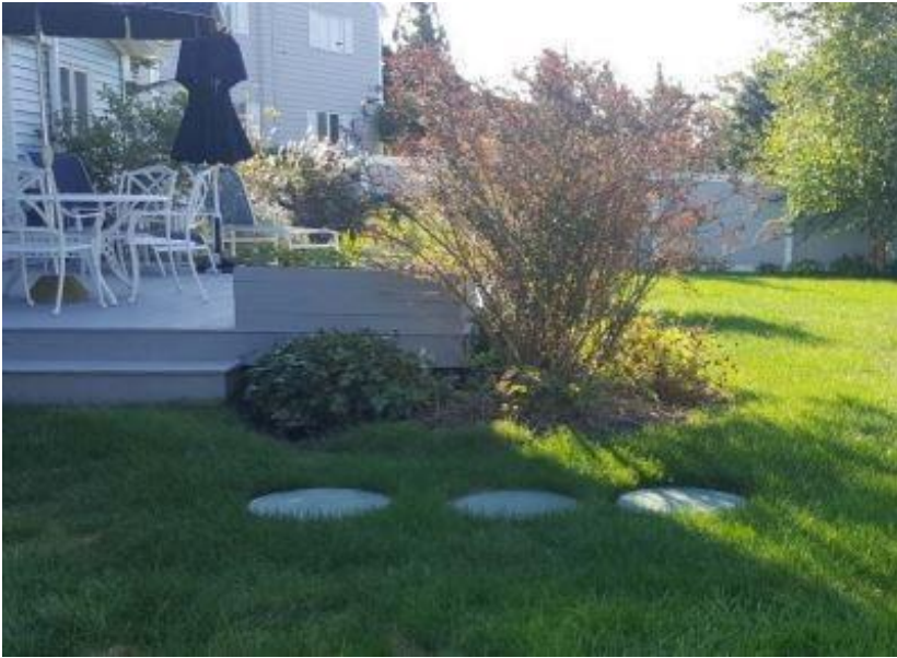
Innovative/Alternative Onsite Wastewater Treatment System Installation (Fuji Clean CEN Series) – Photo Credit: Suffolk County
