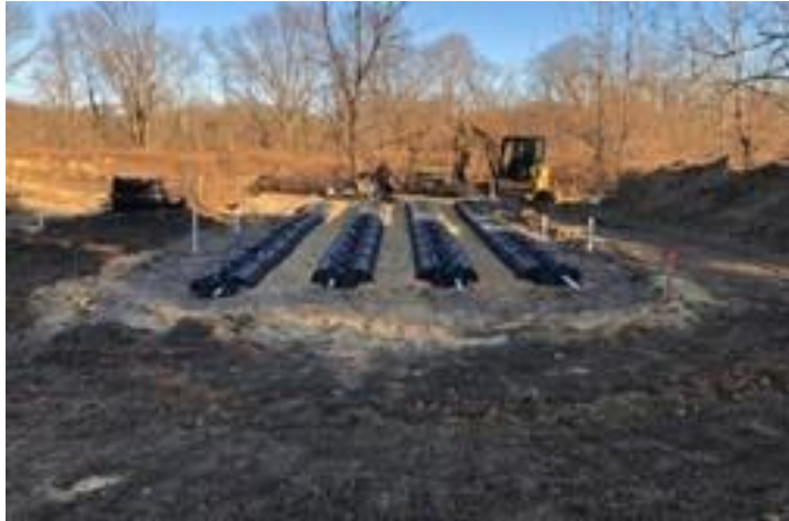
Nitrogen Removing Biofilter. Photo Credit: Center for Clean Water Technology
