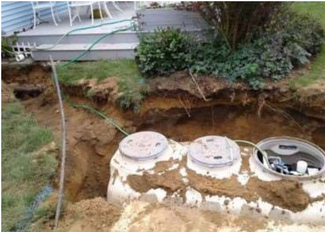
Innovative/Alternative Onsite Wastewater Treatment System Installation (Fuji Clean CEN Series) - Photo Credit: Suffolk County
