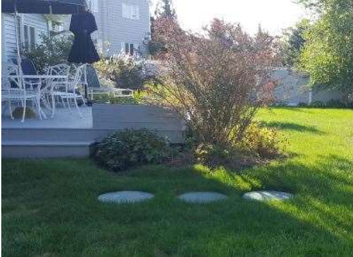
I/A OWTS installed. Photo Credit: Suffolk County
