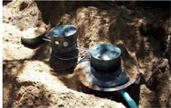
Installation of Hydro-Action system in Nesconset - first I/A OWTS to receive provisional use approval
