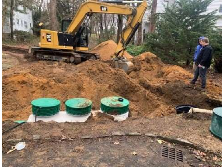
Installation of I/A OWTS at a residence in Manhasset. Photo credit: NCSWCD.
