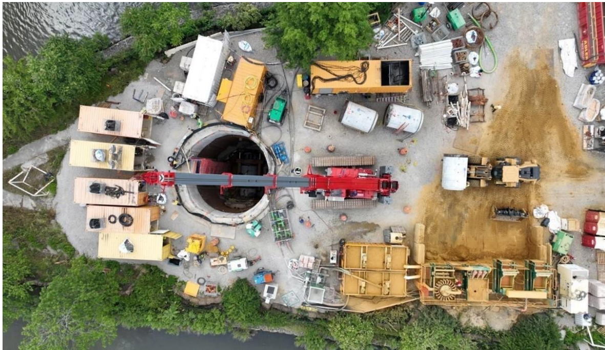
Microtunneling technique used to install piping deep into the ground. Photo credit: DEC
