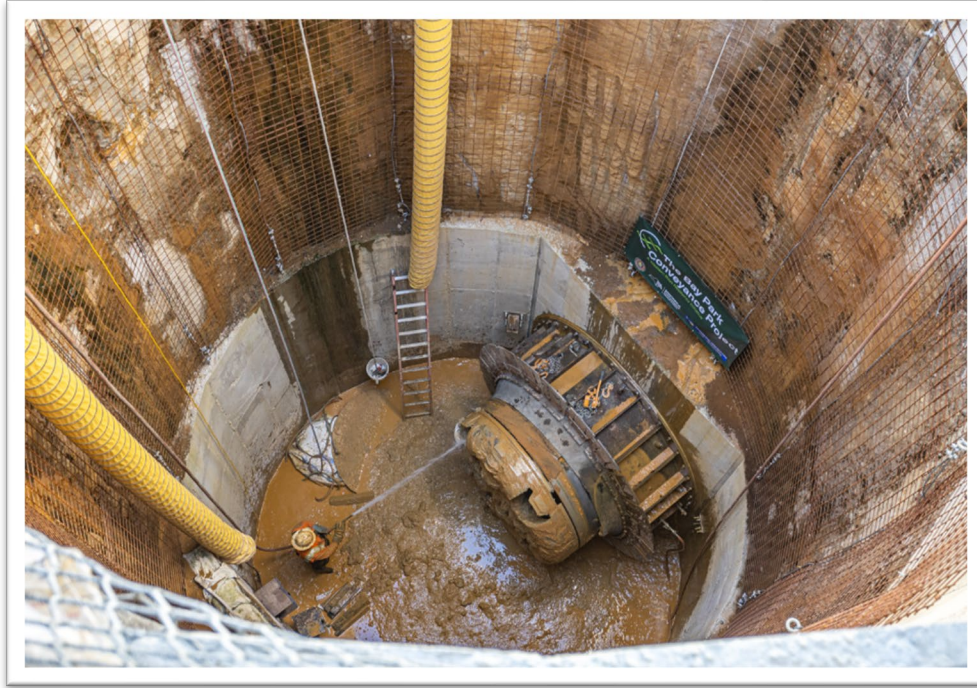
Micro tunneling technique used to install piping for the Bay Park Conveyance Project. Photo credit Nassau County
